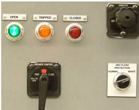
Fig. 3. Breaker control with maintenance switch
