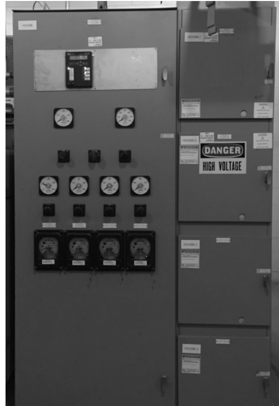
Fig. 3 Manufacturer A Switchgear
