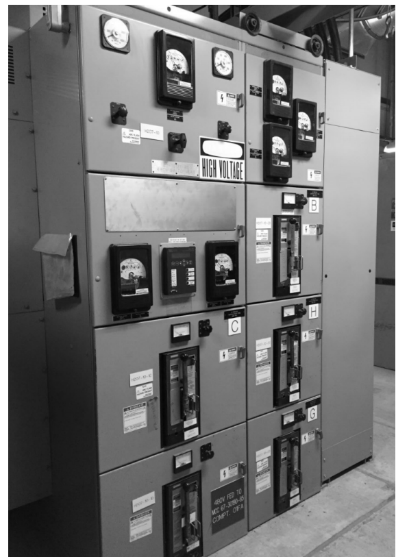
Fig. 4 Manufacturer B Switchgear
