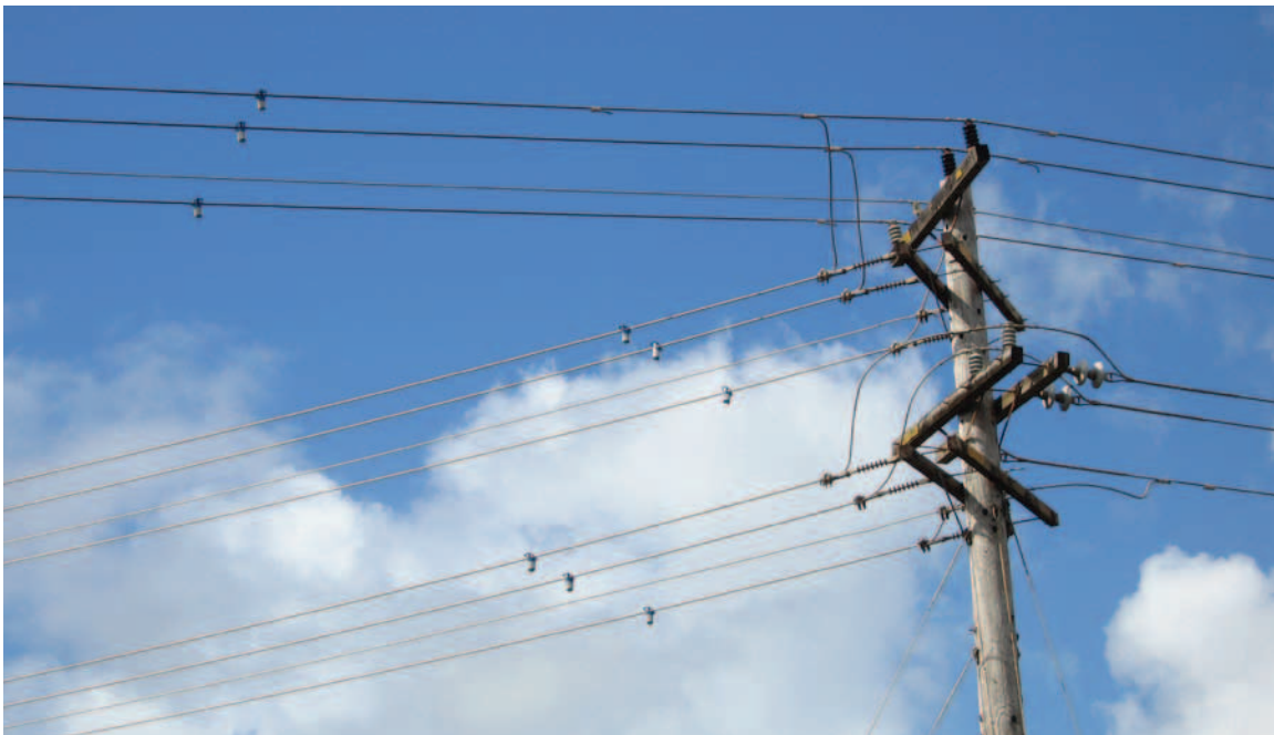
These lucky overhead fault indicators reduce fault finding time in Hawaii.
