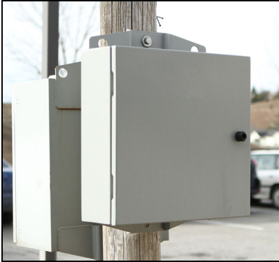
Fig. 9. Pole-mounted field cabinet
