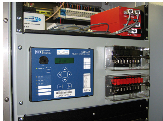
Figure 3—Shown above is a metering and communications cabinet providing secure serial and IP connections for real-time billing metering data, distribution SCADA, load management, and AMR traffic.
