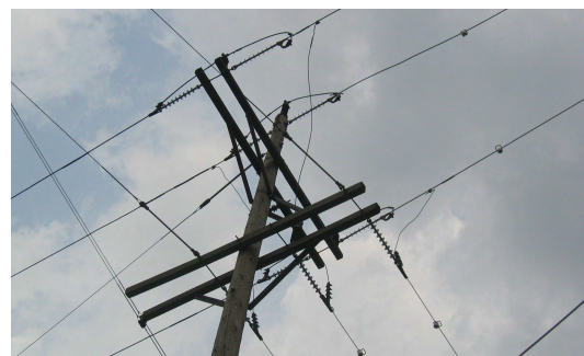
Figure 3—During 2004, 2005, and 2006, We Energies installed SEL ERL fault indicators such that approximately one-third of the company's overall feeders were populated by 2006.
