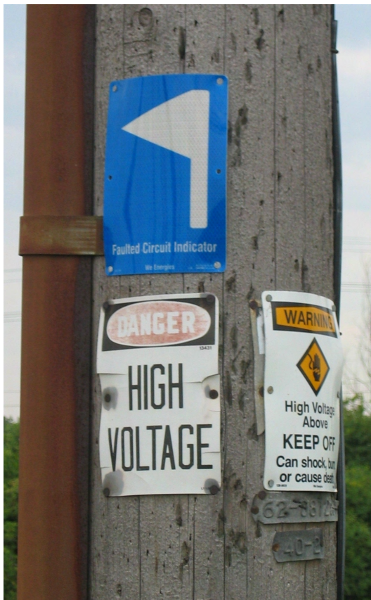
Figure 4—We Energies developed blue fault circuit indicator signs for installation at the base of the pole to identify the location of fault indicators.
