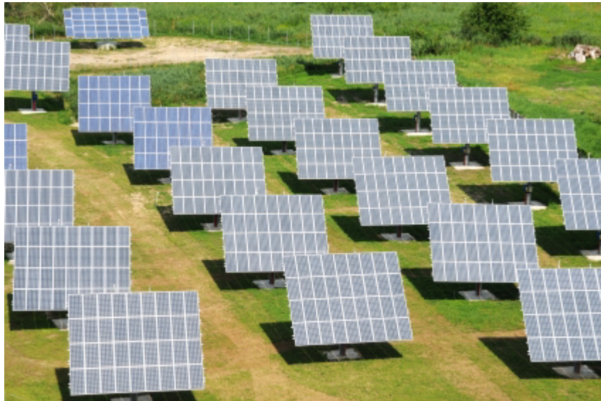
Figure 1 Solar Photovoltaic Arrays
