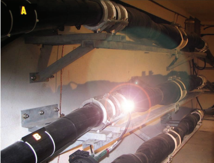
Monitor underground splice applications using a short-haul multimode (MM) fiber application, up to 250 meters.
