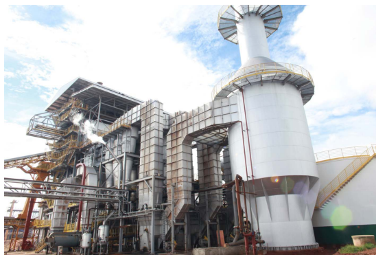
Cargill's new steam boiler plant for sweetener and starch production in Uberlândia, Minas Gerais (MG), Brazil.
