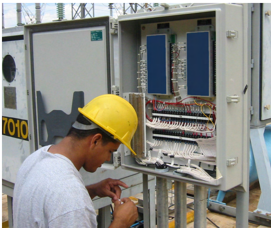
Fig. 5. I/O modules in the yard
