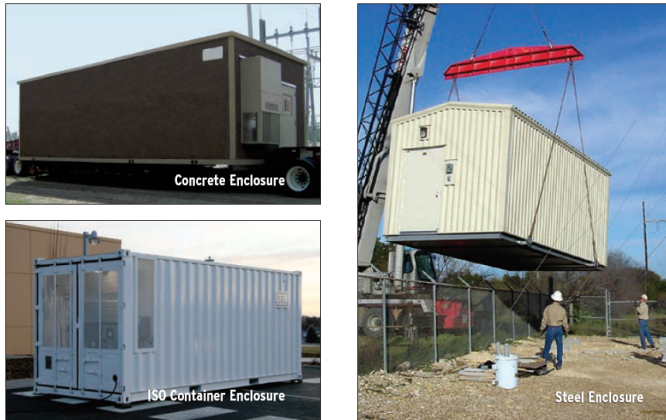
Fig. 12. Substation control enclosures
