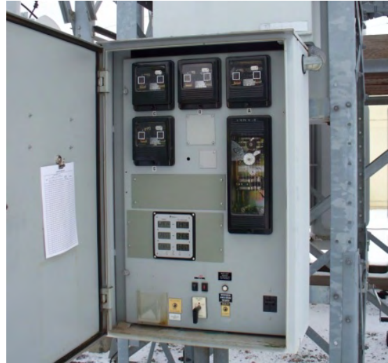
Fig. 3. Electromechanical relays in the yard
