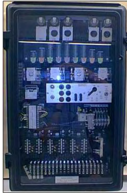
Fig. 30. First generation (electromechanical) protection relay
