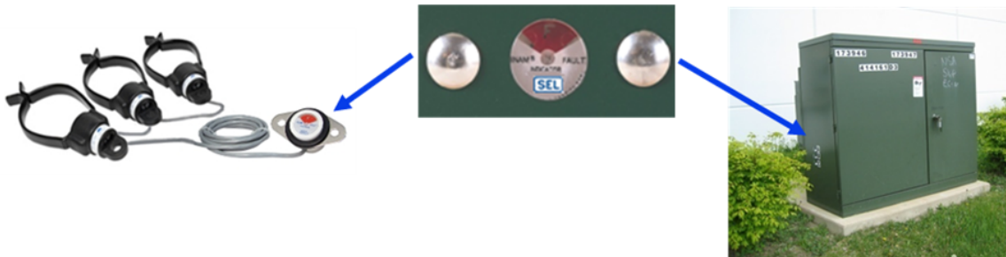
Figure 3 Typical Test Point Reset Installation
