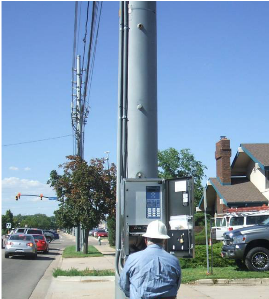
Figure 2 The SEL-651R provides protection and control for inertia reclosers at IPP sites
