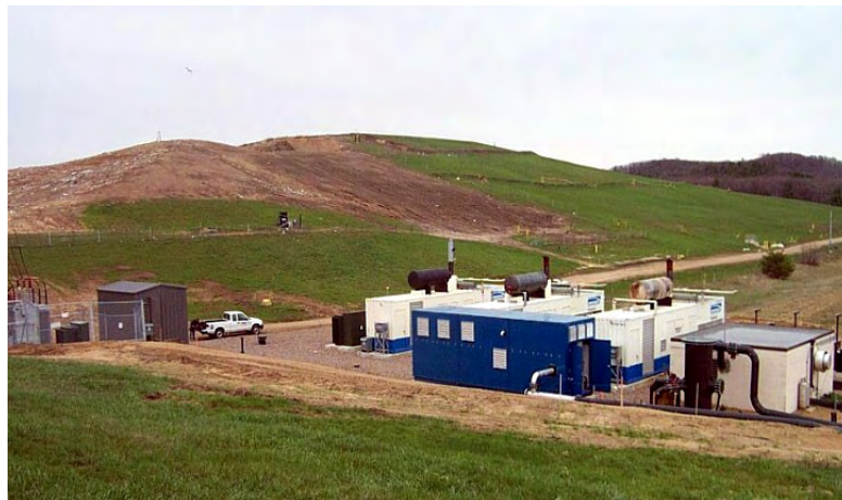
Figure 1 Generators Produce Energy With Surplus Methane
