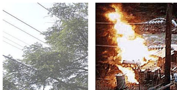
Fig. 5. Trees near distribution lines and a power transformer after an explosion
