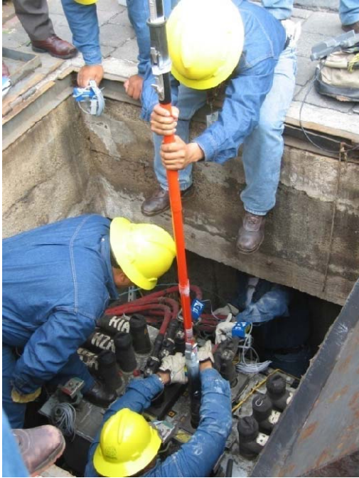
Fig. 2. CFE crews install fault indicators and wireless interface units in Guadalajara vaults
