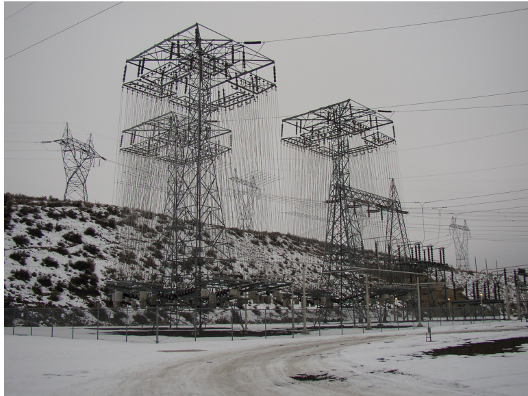
Figure 22 1400 MW Dynamic Brake at Chief Joseph Substation (K. E. Martin photo)
