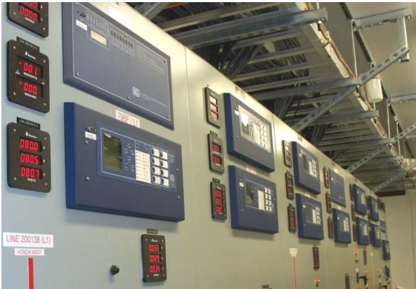
Fig. 1. Relays With Synchrophasors in Protection Panels
