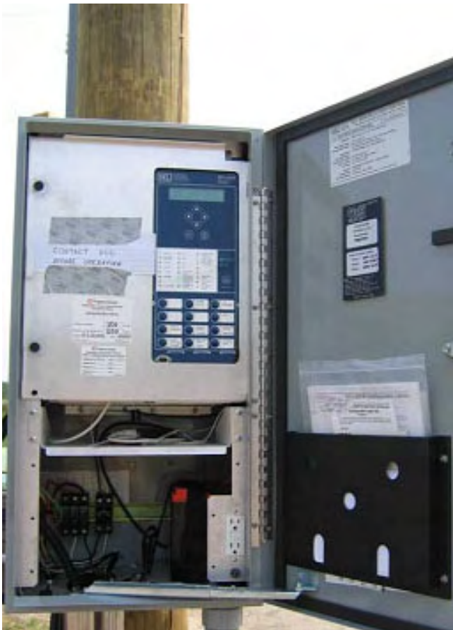
Fig. 5. Advanced recloser control at the interconnection site
