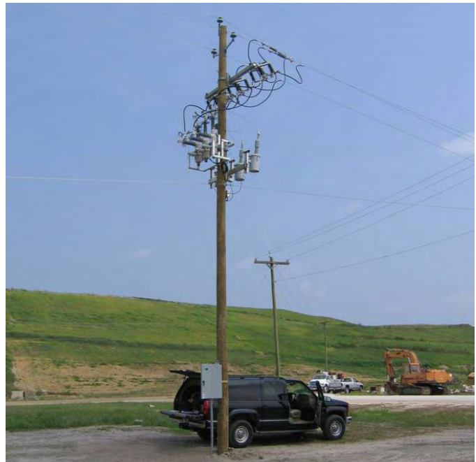
Fig. 4. Intertie recloser installation at IPP site. On the right side of the pole are three 1 kVA PTs monitoring utility voltage. To the left of the pole, the next structure is the IPP point of demarcation and the connection point to underground cables leading to the IPP.
