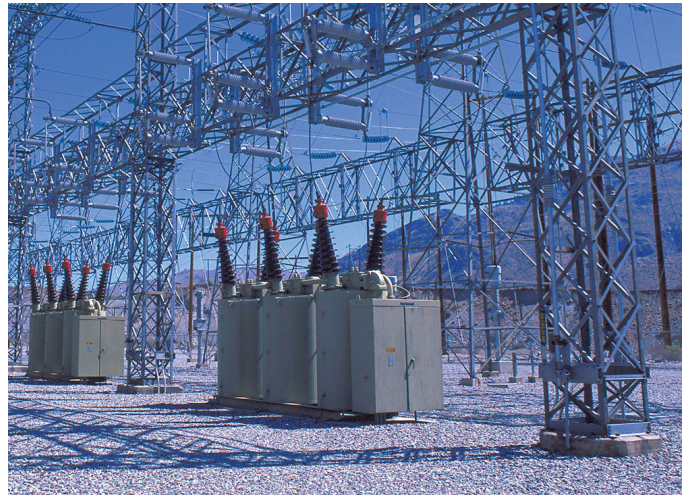
Fig. 1. Utilities need a skilled workforce to support the power system
