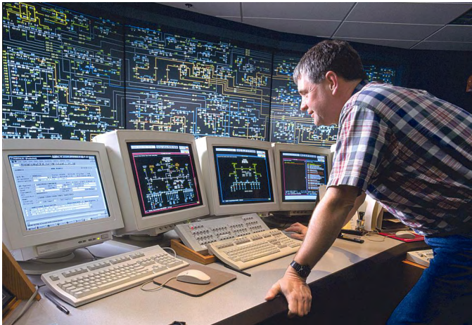
Fig. 4. Typical SCADA console user unaffected by choice of protocol within the substation
