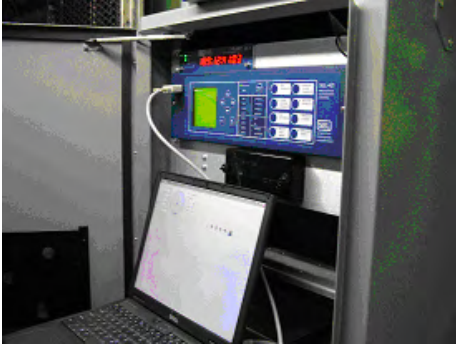
Fig. 8. Relay Providing Phasor Measurements
