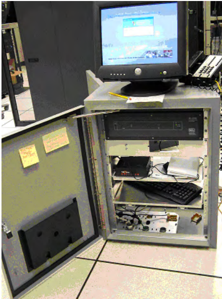
Fig. 10. Phasor Data Concentrator Cabinet in Temporary Location
