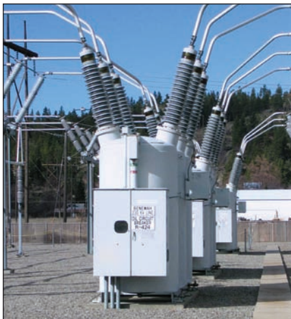
Monitor circuit breaker operating characteristics and history to optimize maintenance schedules.
