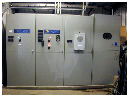
Figure 3—Among the main concerns about integrating the Peter Brotherhood generator with the rest of the waste-to-energy system were the protection, monitoring, and interfacing issues. SEL-300G Generator Relays were purchased to provide the necessary protection for the refurbished generator.
