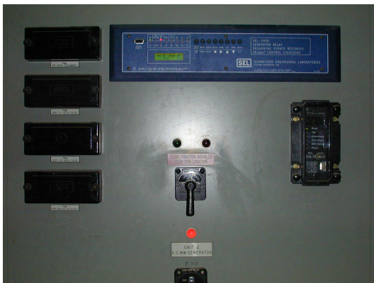
Figure 4—The SEL-300G Relay (shown here installed), the first microprocessor-based technology to comply with IEEE turbine protection standards, includes several unique features designed for unsurpassed protection, monitoring, and control of electrical generators in utility and industrial applications.
