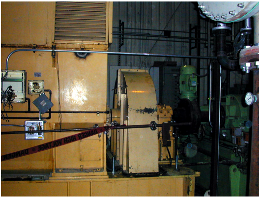
Figure 2—In order to make the transformation as cost-effective as possible, Barlow decided to incorporate a used turbine generator system, which was purchased from a utility in Bermuda.
