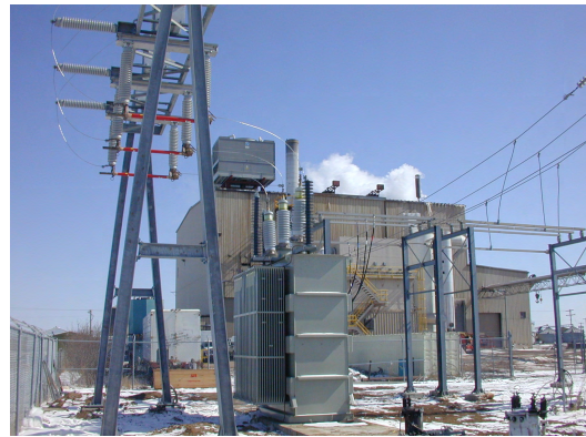
Figure 1—For its second WTE project, in August 2002, Barlow undertook the conversion of an existing trash-burning facility in Perham, Minnesota to a Barlow Aireal-based steam-and-electricity generating plant.
