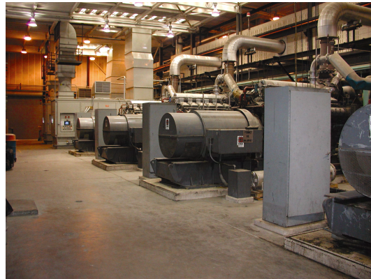
Figure 1—NEI Electric Power Engineering first introduced Metro Wastewater Reclamation District to SEL products in the cogeneration section (shown above) of the Metro plant. The anaerobic digestion process used to produce biosolids also produces methane, which was used to fuel four large electrical generators and heat the ten anaerobic digesters as well as provide electrical power and heat to other buildings on the plant site. Most of the electrical power was sold to Public Service of Colorado, generating about $1.6 million in revenues per year. When that contract expired, two new, more efficient gas turbine units were installed.
