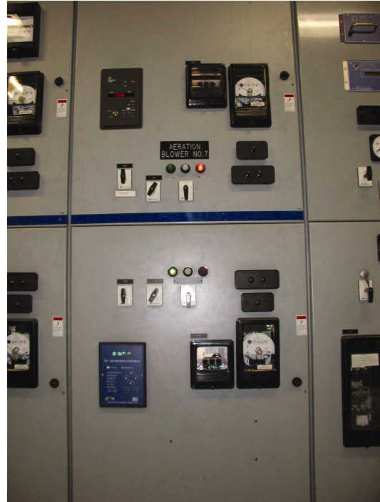
Figure 2—To provide necessary assurance of critical blower system uptime, Metro Wastewater replaced its aging motor protection relays with utility-grade SEL-701 Relays, which offered more durability, robust features, and improved availability at a lower price than conventional relays.
