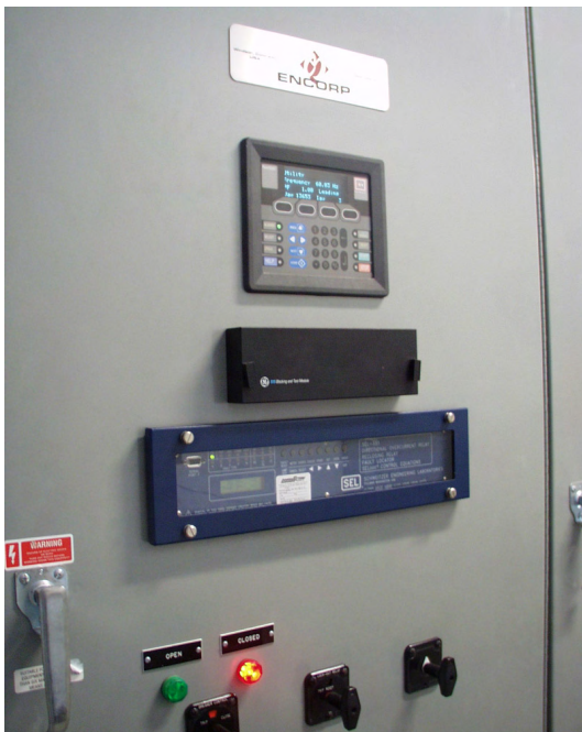
Figure 2—Encorp selected the SEL-351 Directional Overcurrent and Reclosing Relay (shown above) to provide interconnection protection.
