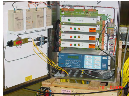
Figure 4—Each switchgear package is equipped with fiber-optic modem/transceiver, current and voltage sensing equipment, and an SEL-351S Protection and Breaker Control Relay.
