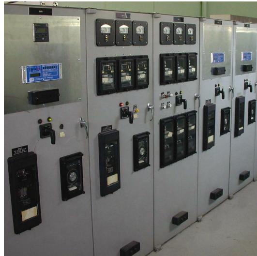
Figure 1—The planning department of ENWIN Powerlines has updated and upgraded its 27.6 kV substations to meet the rigorous requirements for added reliability, protection, and control of the electric power system.
