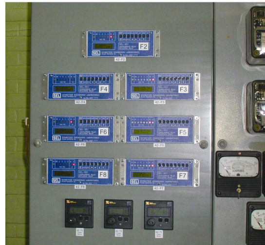
Figure 4—Overloads were not known for weeks with the “old system,” now overload status is instantly recognizable using the relay’s visual alarms. The installation of SEL-551 Relays economizes on space and improves functionality for seven feeders.
