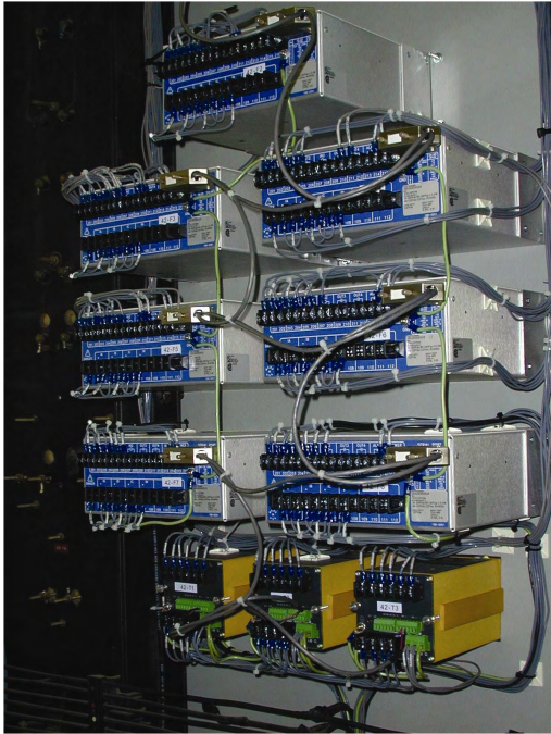
Figure 5—Rear view of the compact installation of protective relays for seven feeders. Simple wiring and control I/O are readily accessible.
