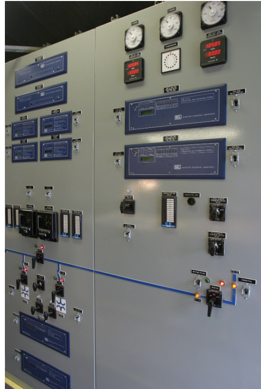
Figure 2—The upgrade of old relays and control panels was completed using relays from Schweitzer Engineering Laboratories, Inc. SEL equipment was preferred because of the array of features available in a single relay, and the fact that SEL equipment meets the "utility grade" requirements of PG&E.
