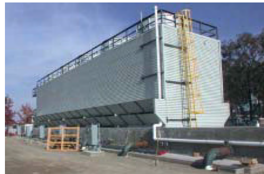
10-MW Cooling Tower
