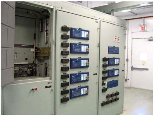
Figure 5—Microprocessor-based relays and other electrical devices are centrally located. Previously, electromechanical relays were used and required one relay per function. With microprocessor-based relays, only one relay is required for multiple functions.
