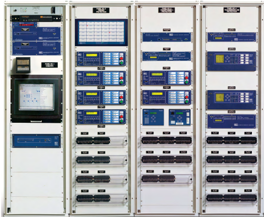
Figure 3—The SEL-7000 Integrated Substation System was installed in a separate communications panel containing communications equipment and the HMI system.
