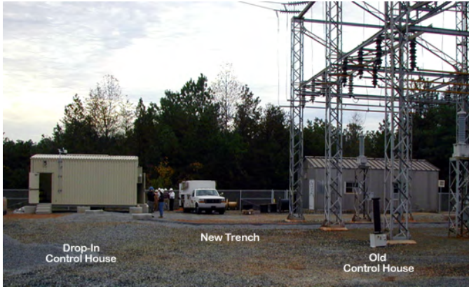
Fig. 2. Old and New Control Houses in Belmont Tie Substations
