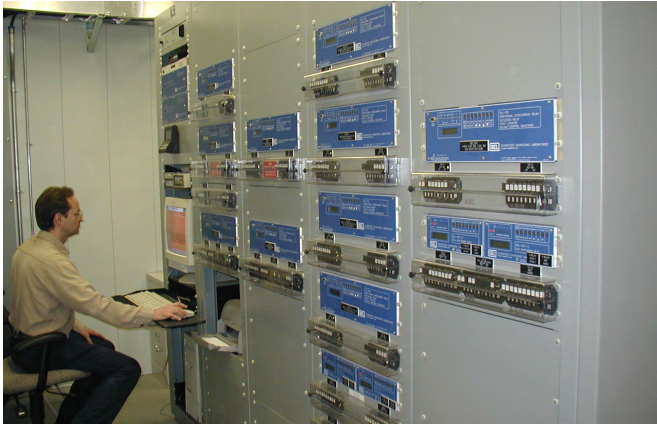
Fig. 3. Panel Configuration Inside Control House
