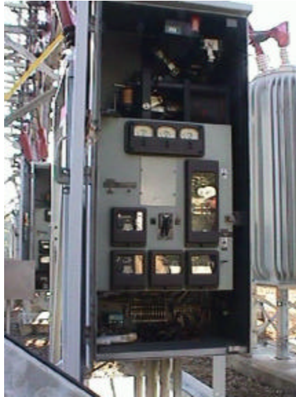
Figure 22 Breaker Control Cabinet with Electromechanical Relays, Meters, Control Switches and Indicating Lamps
