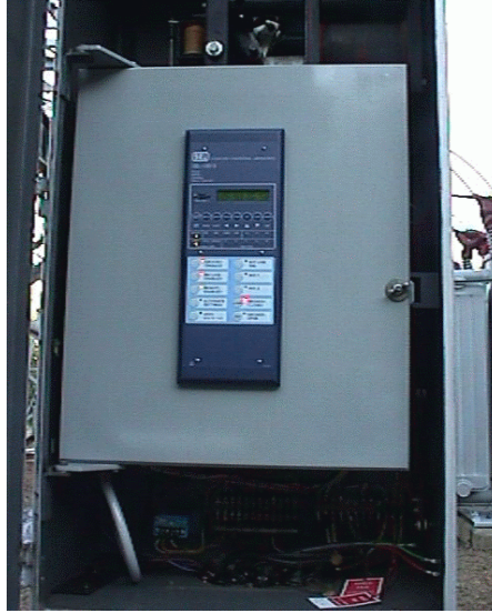
Figure 23 Breaker Control Cabinet with Retrofitted Numeric Relay
