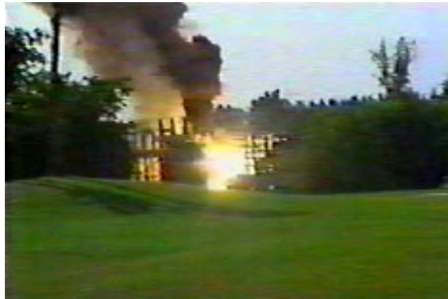
Figure 11 DC Battery Failure Causes Complete Loss of Substation
