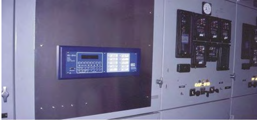
Figure 2 Modern SEL Multifunction Relay and Traditional Electromechanical Design
