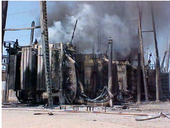
Figure 12 Transformers Destroyed Due to Through-Fault Damage
