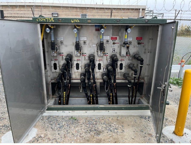
Fig. 1. Inside the Four-Way Pad-Mounted Switch
