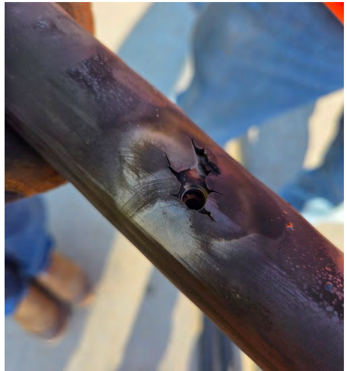
Fig. 2. Damaged underground cable.
