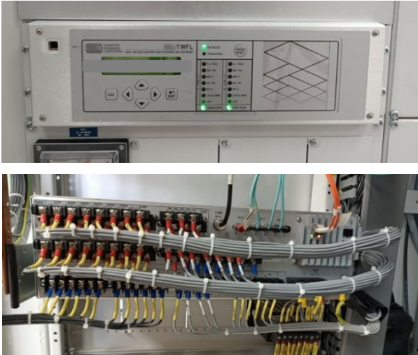
Fig. 12. TW-based device installed on a protection and control cabinet at the Paraiso substation.
