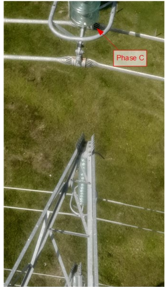
Fig. 32. Bird contamination observed on Phase C at Tower T-424 of Guarayos-Paraíso Line 1.
