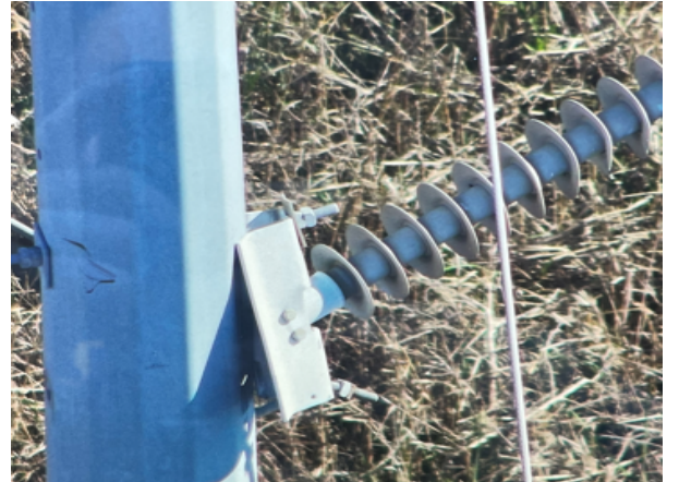
Fig. 4. Picture of Failed Insulator Support
