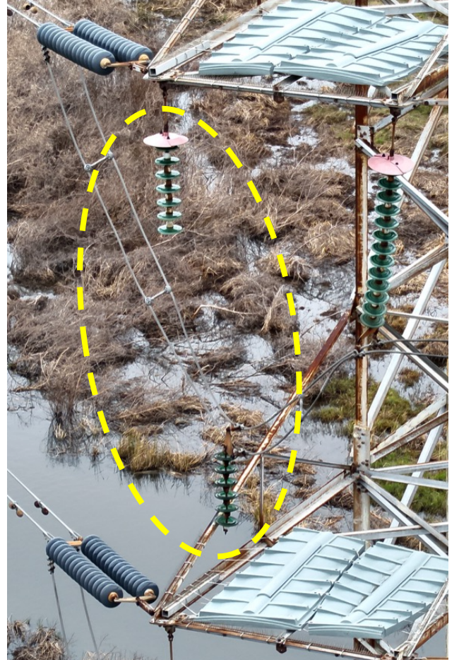
Fig. 10. Suspension Insulator Broken in Half
