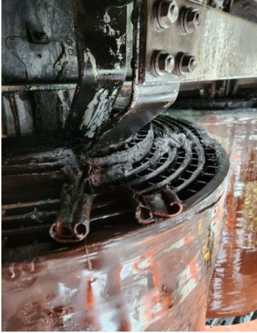
Figure 2 Damage Due to Second Failure
