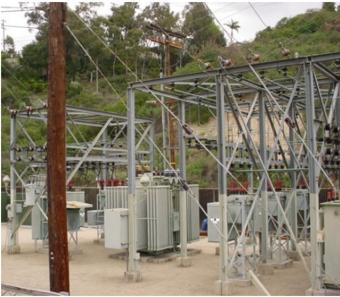
Fig. 3 Older 4 kV substation equipment ground view
