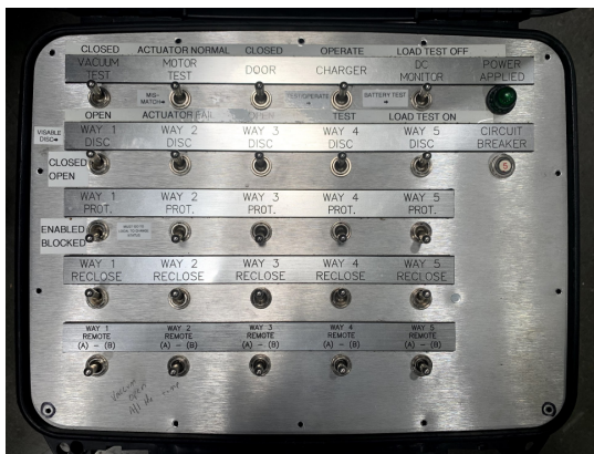
Fig. 24 PLC control panel with toggle switches
