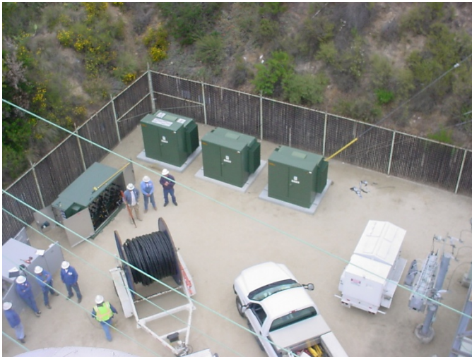
Fig. 4 Substation with new switchgear design
