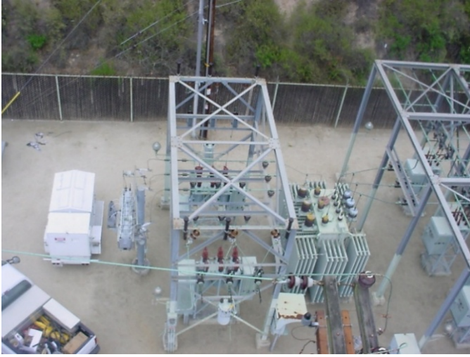
Fig. 2 Older 4 kV substation equipment overhead view
