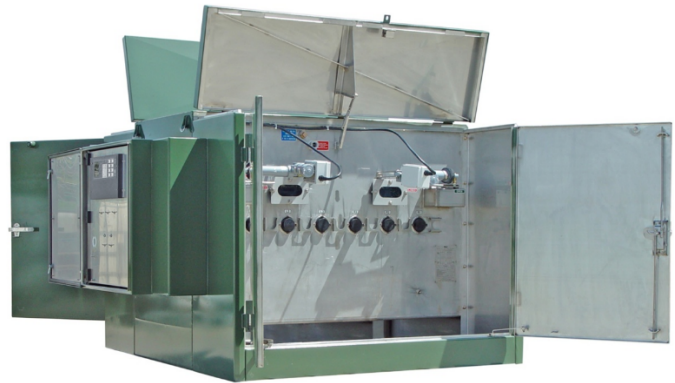
Fig. 1 Example of a pad-mounted switchgear cabinet used by SDG&E
