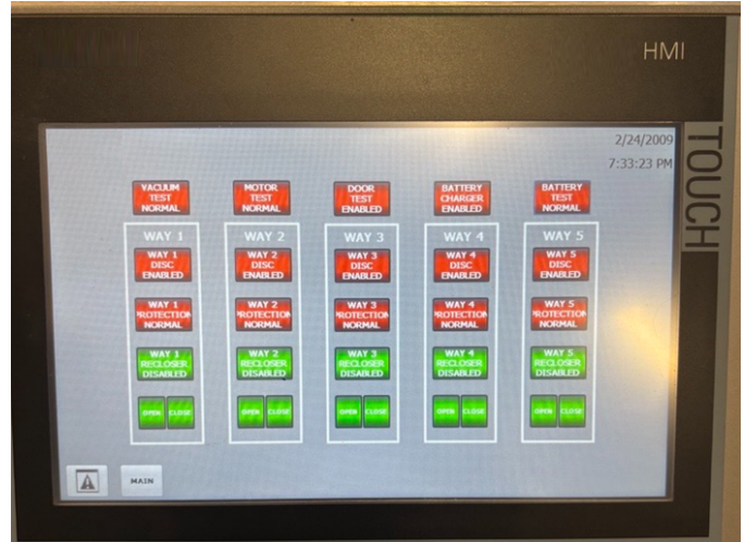
Fig. 25 PLC control panel on touchscreen
