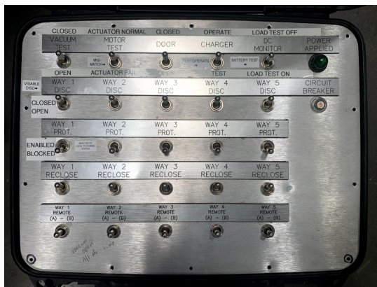
Fig. 24 PLC control panel with toggle switches
