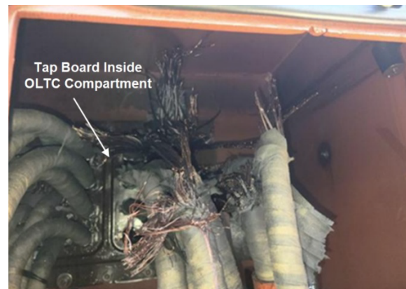
Fig. 4 Cable Failure at OLTC Tap Board on Bulkhead
