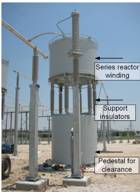
Fig. 1 Air-core series reactor installed at 138 kV substation
