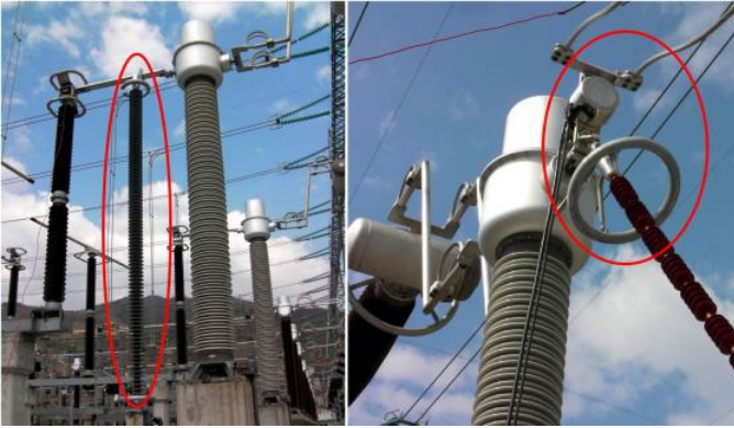
Fig. 1. OCT installation example at Chicoasén, Mexico.
