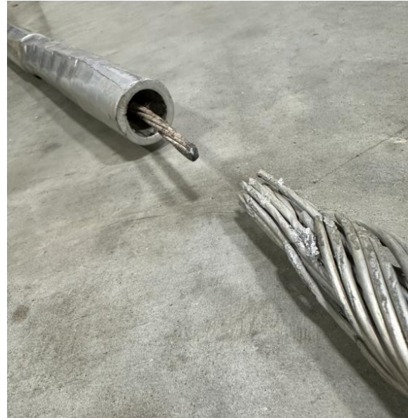
Fig. 4 Splice failure of the 115 kV line.
