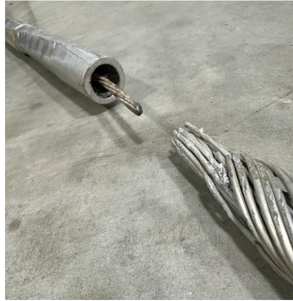
Fig. 4 Splice failure of the 115 kV line.
