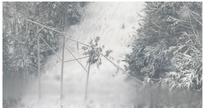
Fig. 10. A tree contact was the cause of the fault shown in Fig. 9 (photograph and fault records courtesy of Puget Sound Energy).
