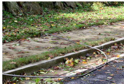
Figure 1 HIF Caused Due to a Downed Conductor
