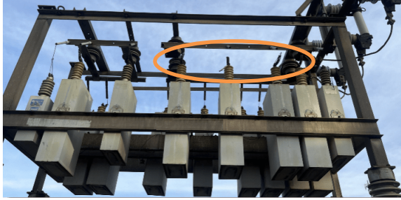
Figure 14 Blown Fuses on the Capacitor Bank
