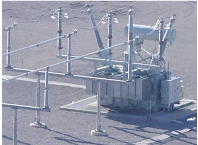
Fig. 1 Ameren 345 kV liquid-immersed gapped iron-core reactor.
