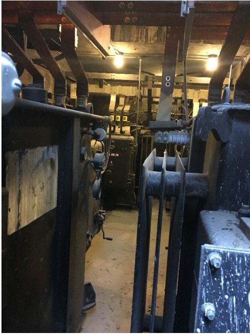
Fig. 6. Inside a small 480 V network vault.
