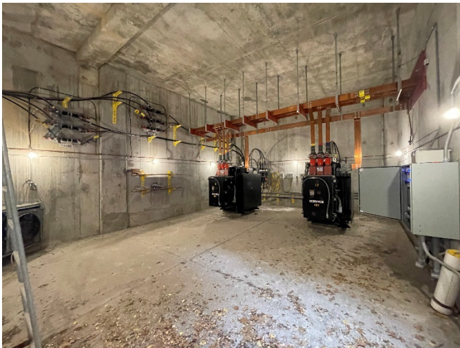
Fig. 7. Inside a large 480 V network vault.
